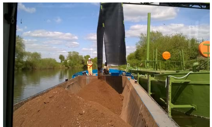
Loading sand and gravel onto a barge at Ryall's Court Farm Quarry
