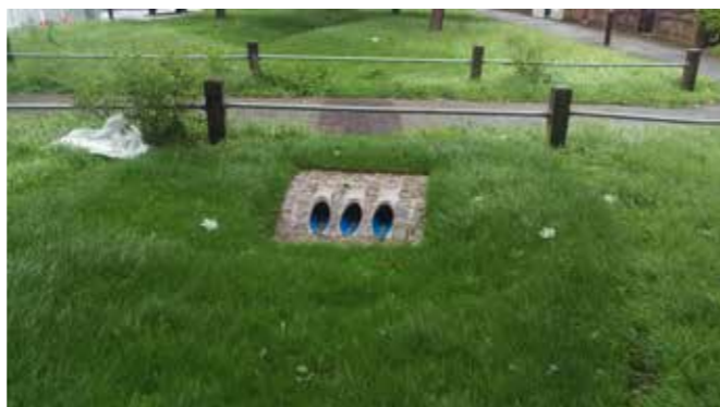
Concrete pipe surround has been used here to provide minimal cover for a driveway crossing at Devonshire Hill, Haringey.
