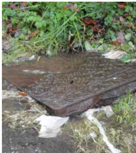
Sewer Flood © Severn Trent Water
