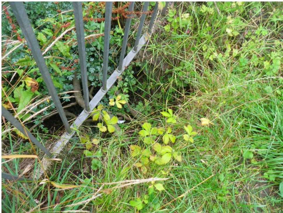
Photograph 12 - Flood defence at Paper Mill, Brooklands Lane, showing bank erosion
