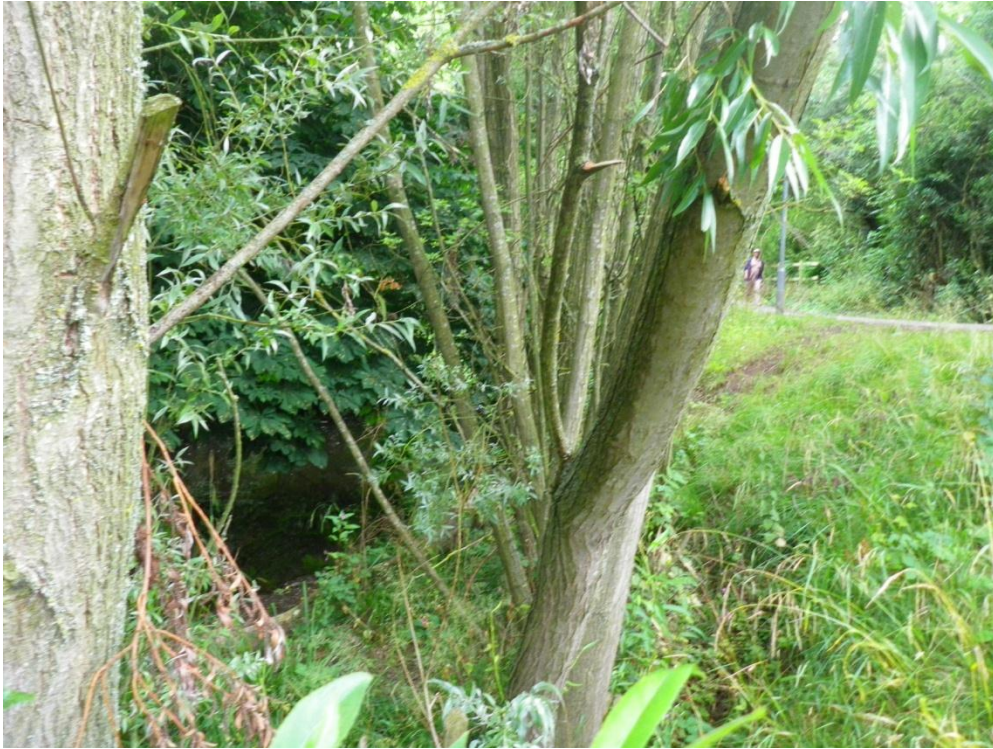
Photograph 11 - Flood defence at Paper Mill, Brooklands Lane, showing bank erosion
